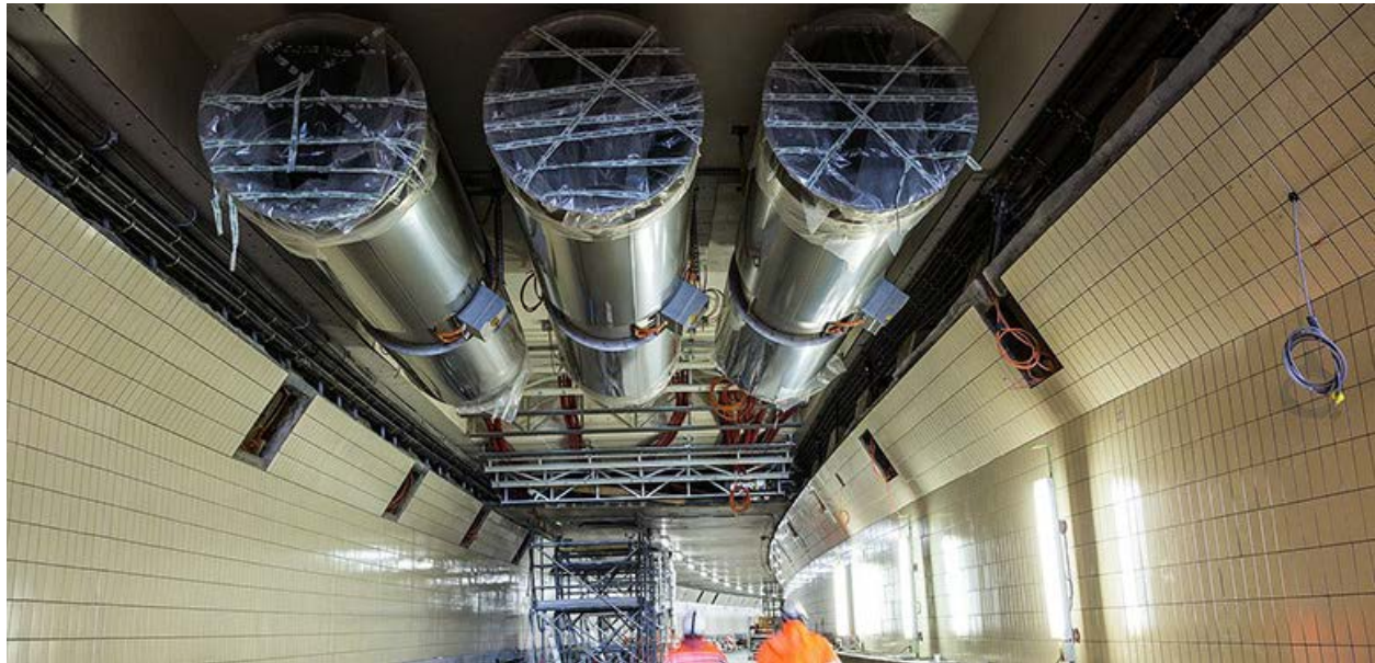
Figure X New mechanical systems that form part of the retrofitting of the Maastunnel currently underway 54 .
