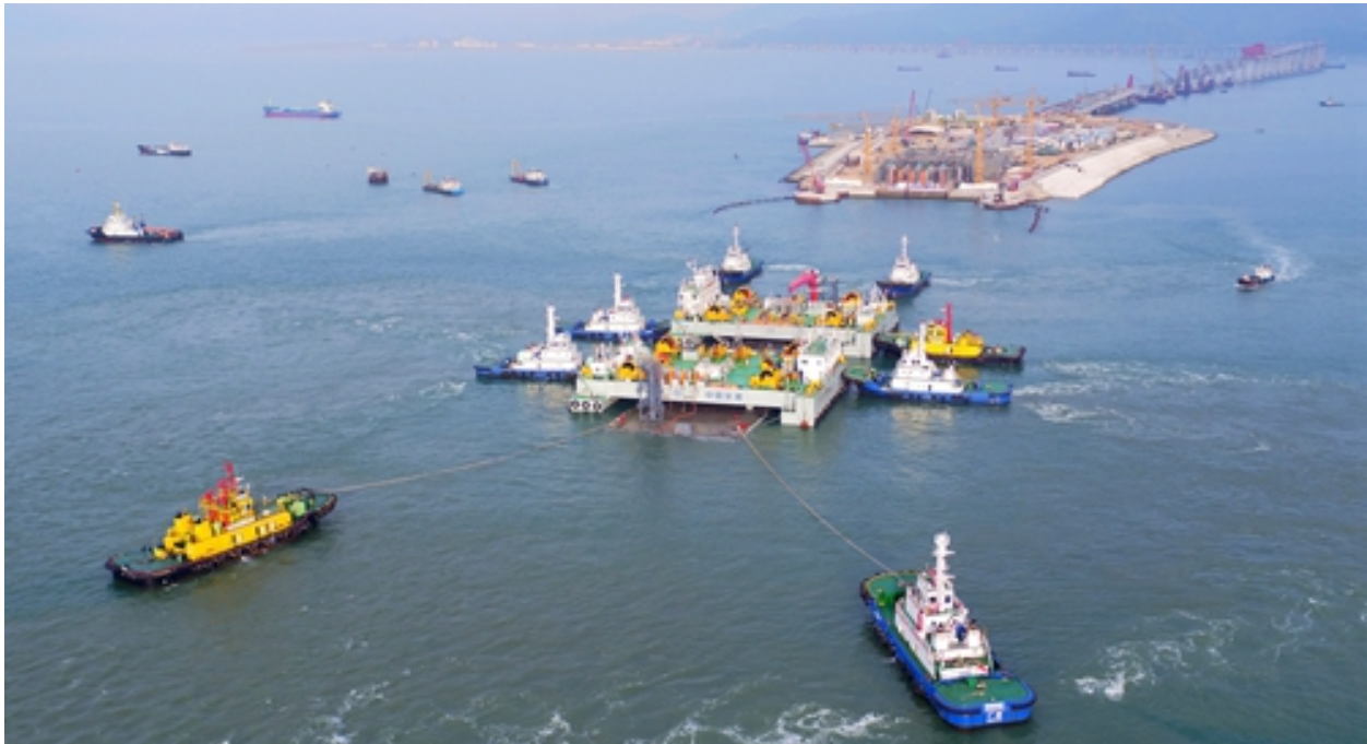
Figure DD Tunnel element being placed in a busy navigable channel for the Hong Kong Zhuhai Macao Link in China 62 .
