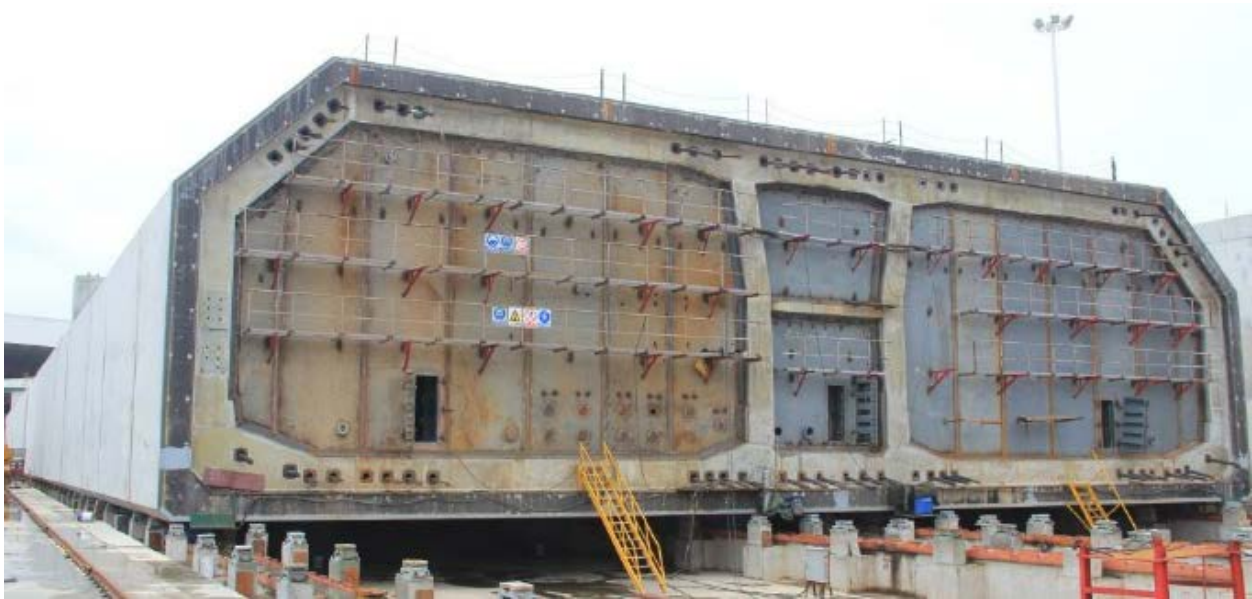
Figure FF Tunnel element being fabricated for the Hong Kong Zhuhai Macao Link in China 63 .
