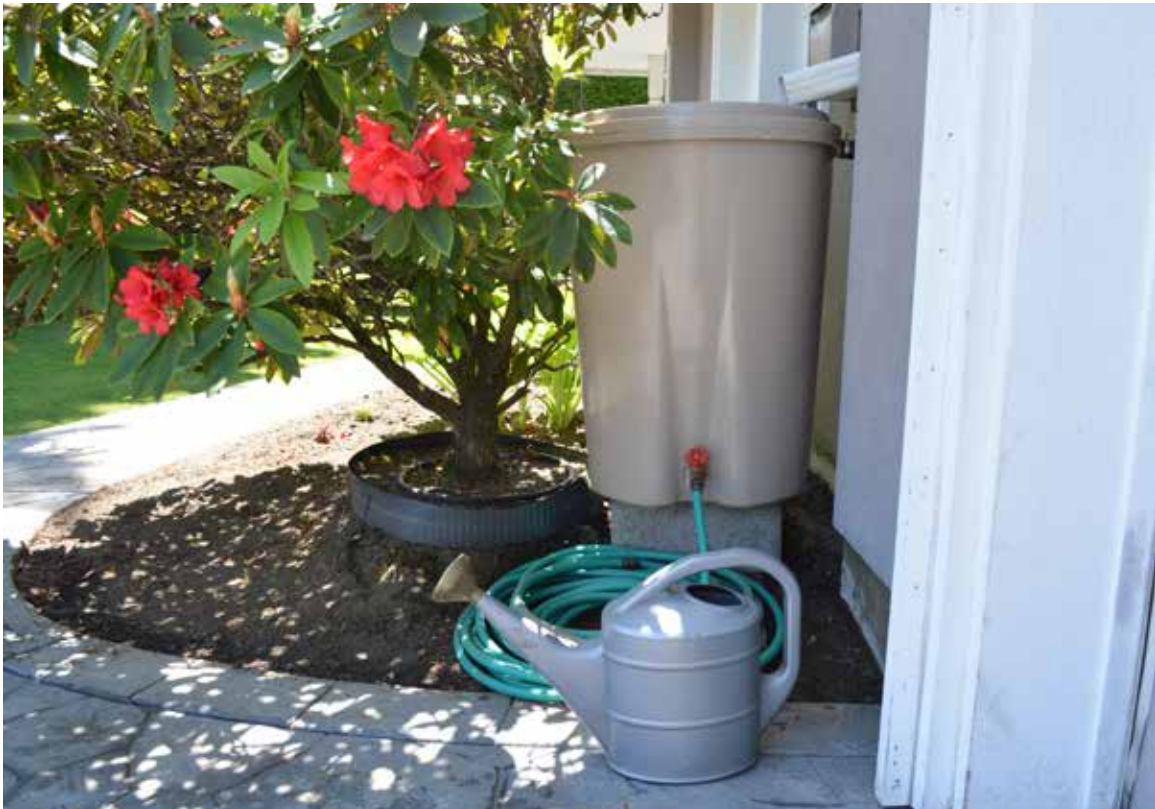
Rain Barrel Connected to Roof Spout and Hose
