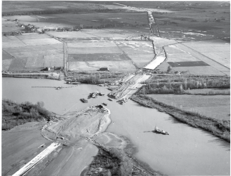
City of Richmond Archives photograph 1984 3 1, taken in 1958, shows the construction of the freeway just south of the George Massey Tunnel. The photo is on page 149.
